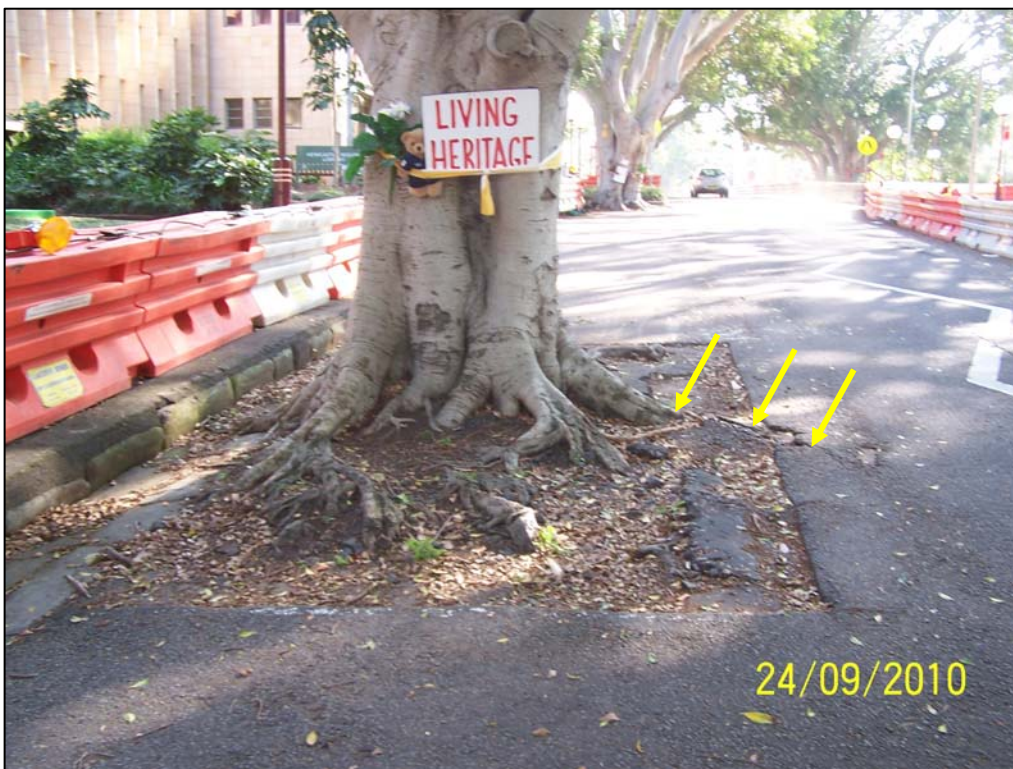
Figure 7 Lifting and cracking of the relatively new layer of bitumen indicating root presence from a buttress (tree 12021).
