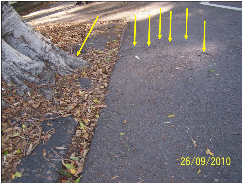
Figure 6 Lifting and cracking of the street surface indicate the presence of roots extending from the buttress of tree 12020.
